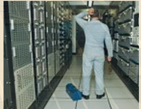
Server and communications facility
