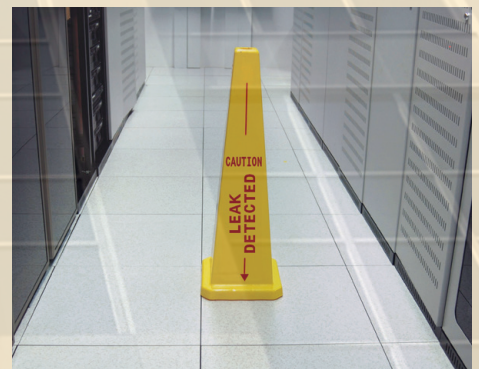
Raised floor computer facility
