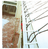
Snow Melting and De-Icing
